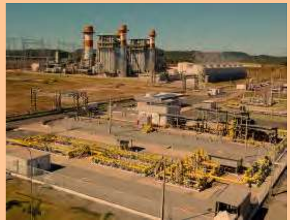
On site: an Eneva facility in Brazil's Parnaiba basin
